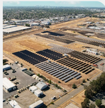
3MW solar array at Depot Park in Sacramento, California, generated 3.750MWhs of solar energy used by Link Logistics in 2022.
